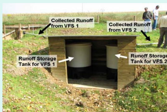
Figure 1. Cutoff walls, Coshocton Wheel samplers (above), and runoff storage tanks for manure plots (below).
