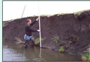
Fig 2. Severely eroded stream bank height and length survey using height pole and tape measure.
