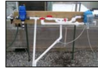
FIG 3 – Chemical injection pumps controlled the dosing process, providing nutrients and treatment to supply laterals.
