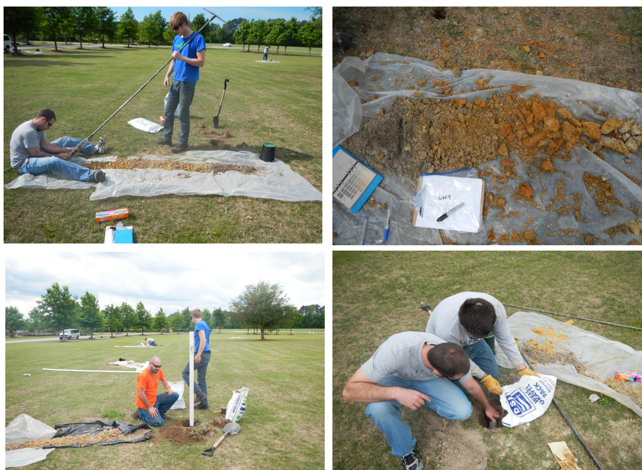
Figure 1. Monitoring wells were installed between the drainfield trenches of the onsite wastewater system. Soil profiles were described and soil samples were collected for particle size distribution analyses. Wells were finished below grade and encased in protective valve boxes.
