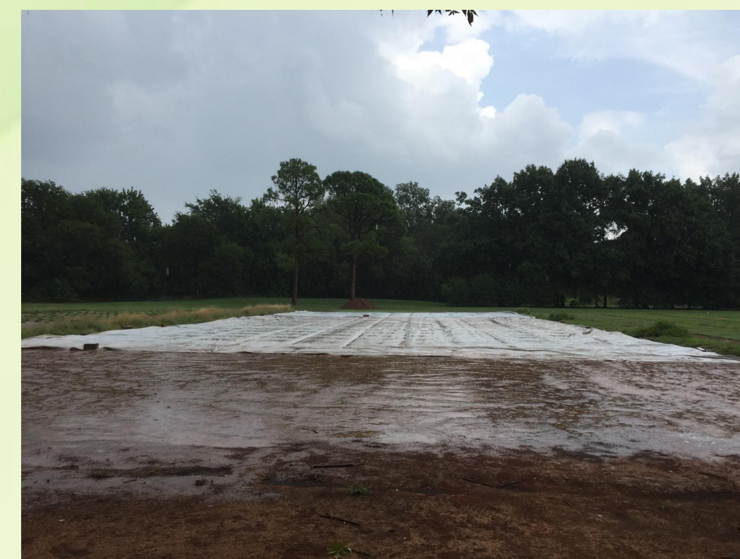
Figure 2. View of Trial 2 being protected by a water proof tarp during a rain event.
